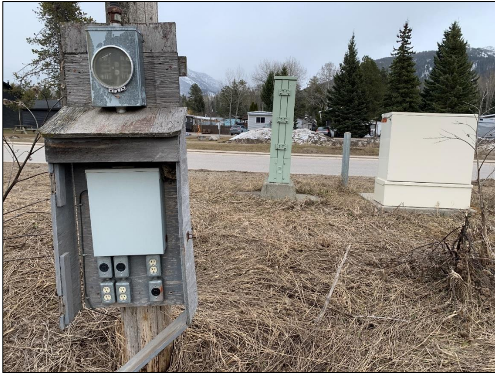
Photo 17: Utility boxes observed along Cokato Road east of the Site.
