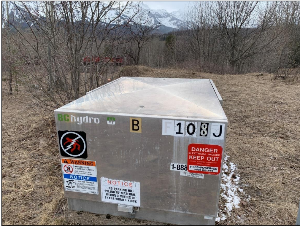
Photo 19: A view of the BC Hydro box observed east of the Site near the other utility boxes.
