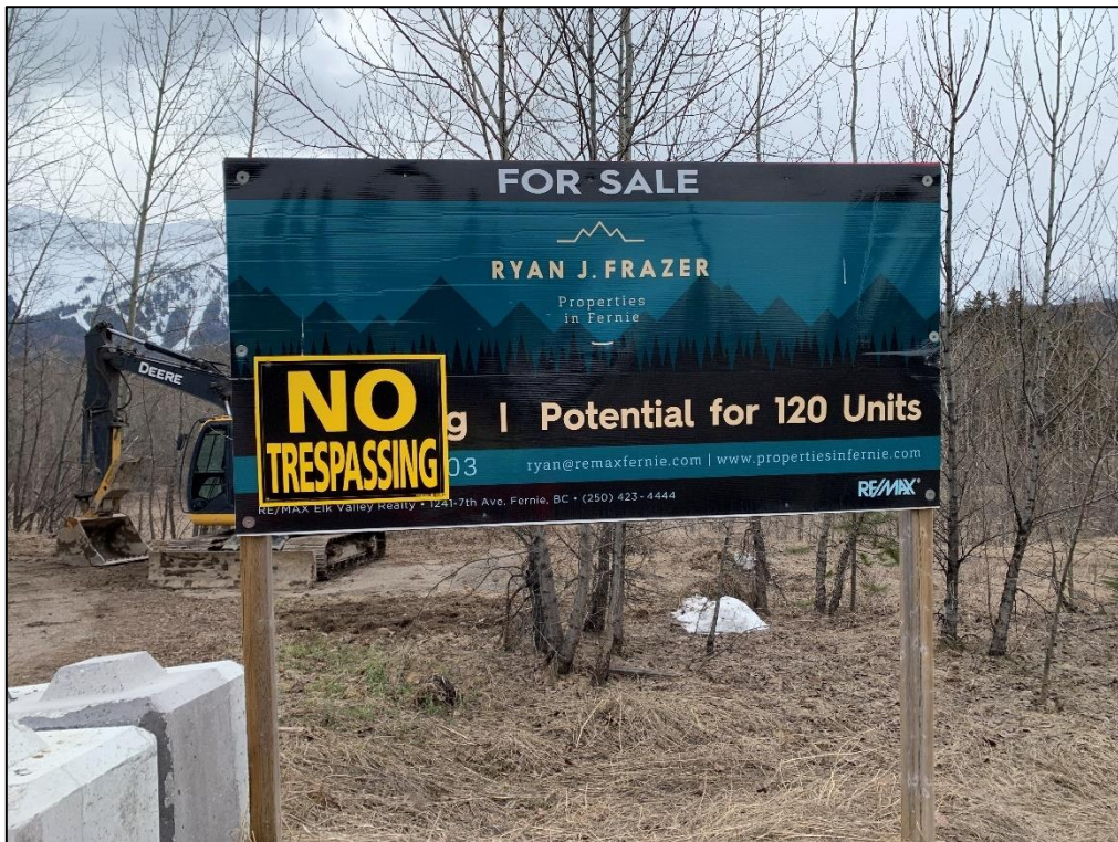
Photo 2: A view of the entrance to the Site and the excavator parked behind the sale sign.
